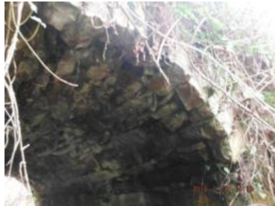
The bridge showing arch separation
